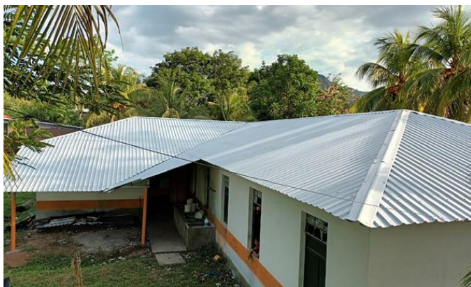
A new roof was recently built for the laundry area near dormitories in Tamagas.
